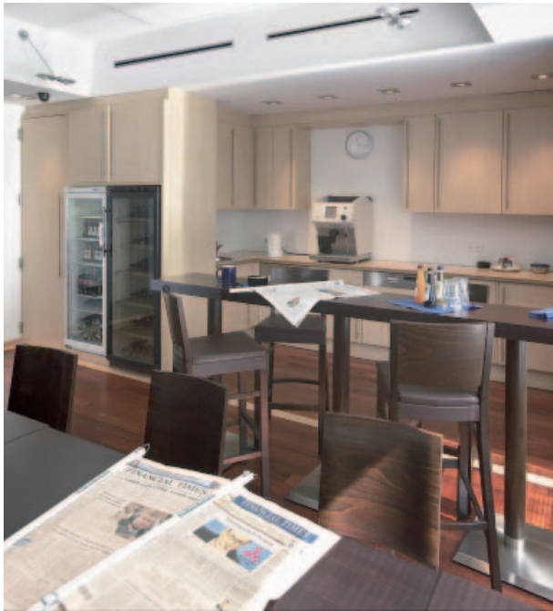
Fig. 2: Wall slot diffuser in the recreation room of an office building
