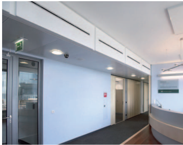
Fig. 3: Wall slot diffuser in the entrance area of an office building
