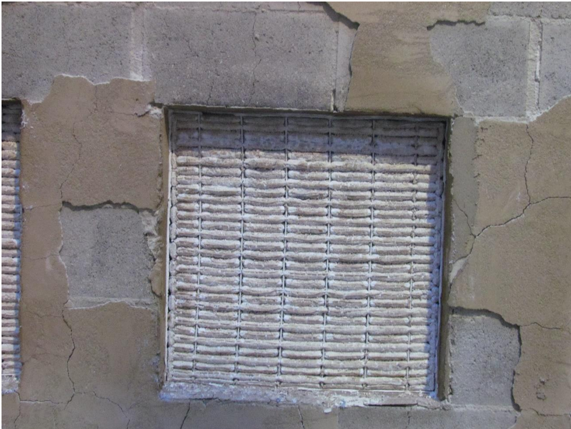
Exposed side after test.
