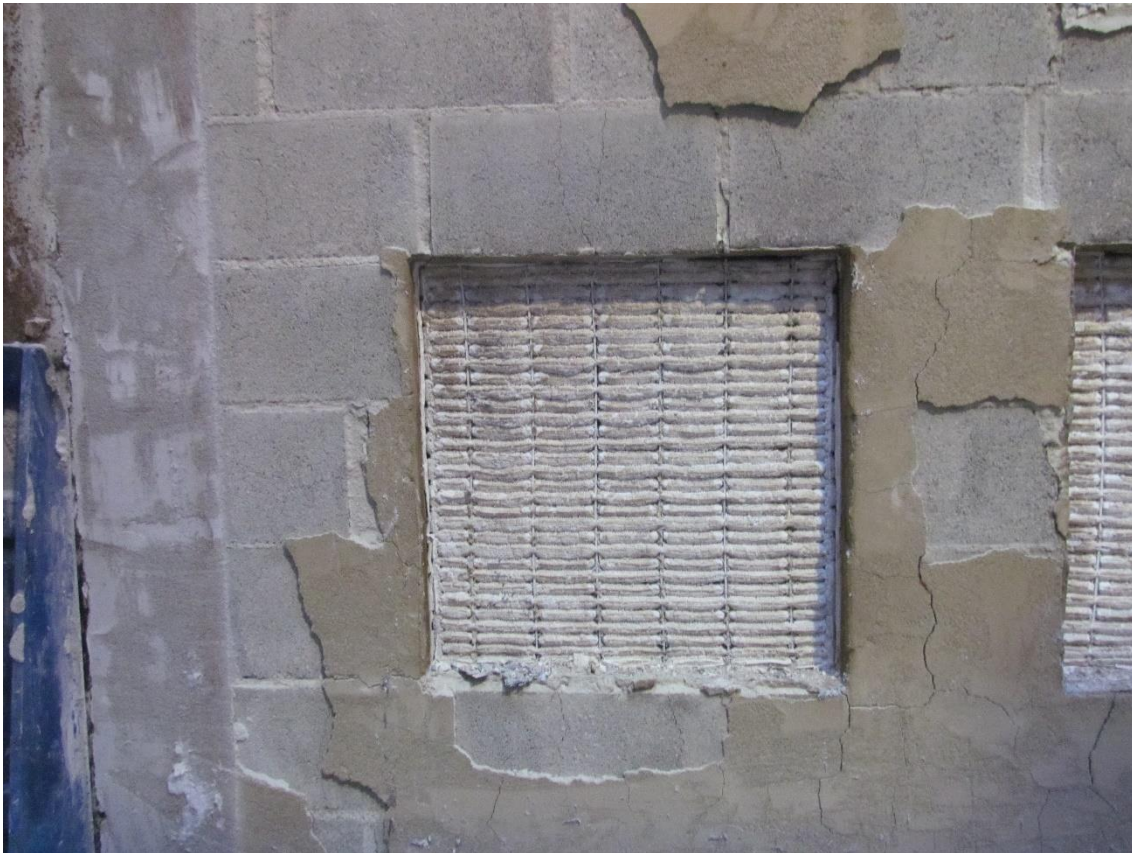
Exposed side after test.
