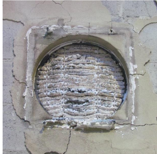
Exposed side after test.
