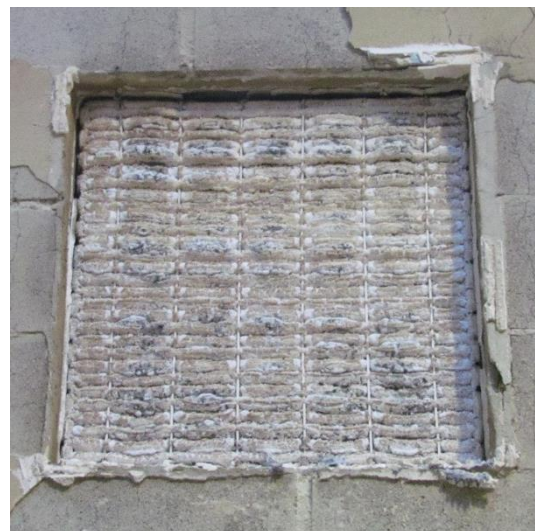
Exposed side after test.
