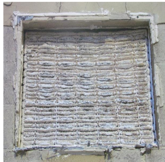
Exposed side after test.
